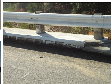
Year built (1939) is stamped on right side of Historic Wardlow Wash bridge curbing. Socketed curb indentations can also be seen.
