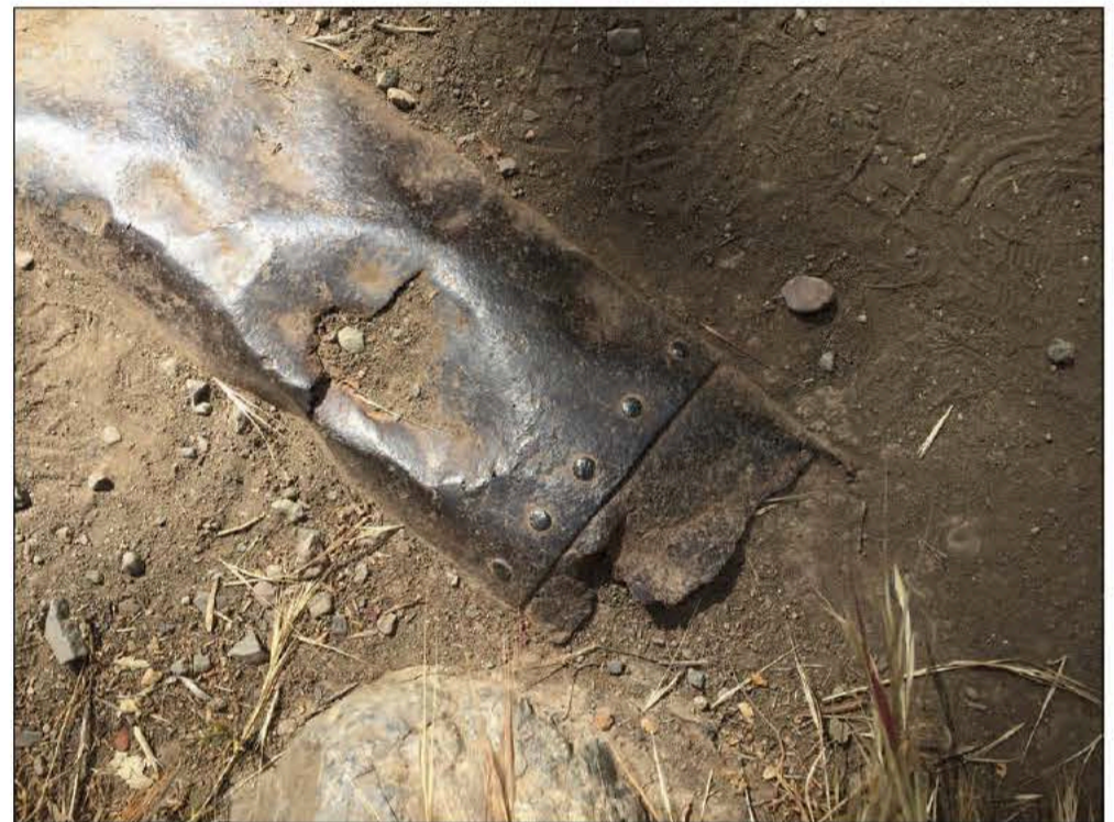
Old abandoned water pipe located in Hagador Canyon
