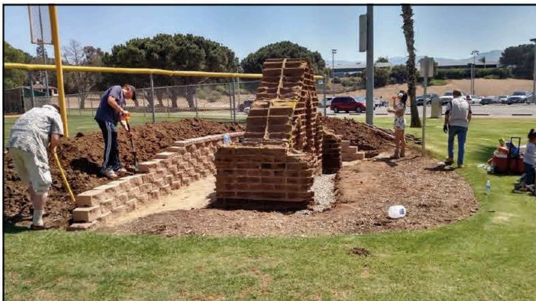
Retaining wall work is in progress at the Veterans Memorial Wall, located at Butterfield Park and dedicated in 1969
